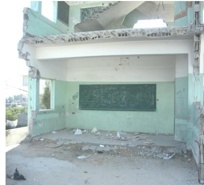
Destroyed wing of a secondary school in Beit Lahiya, Northern Gaza, November 2009
