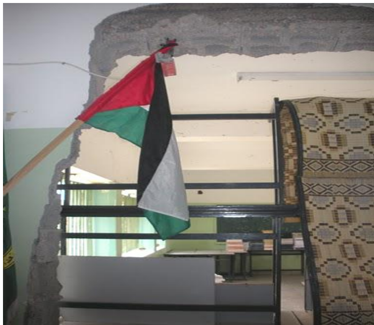
Classroom wall destroyed during the military operations, North Gaza, October 2009.
