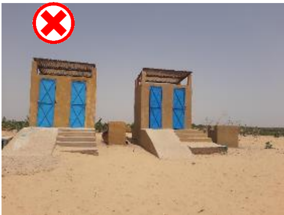
Ramp that is too steep, Fourkoulom, Chad 2022
